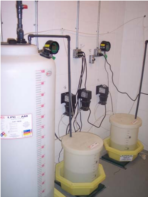
Chemical feed set up for iron and manganese control
