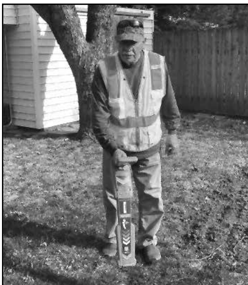
Locating service lines is one of the many tasks Randy undertakes as a Circuit Rider.
