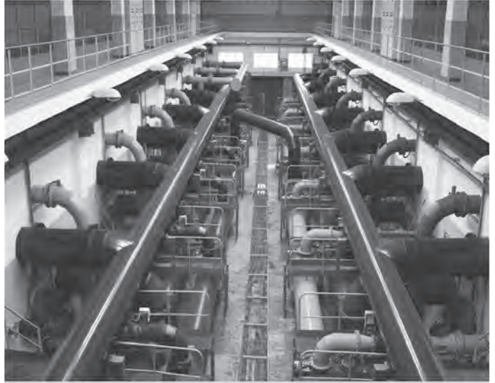
Eliminate Condensation And Manage Humidity In Your Water Treatment Facility with Quest
