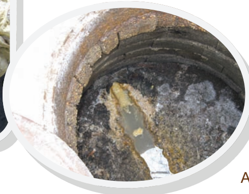
Grease in a sewer manhole
